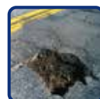
POTHOLE/ DAMAGED PAVEMENT
